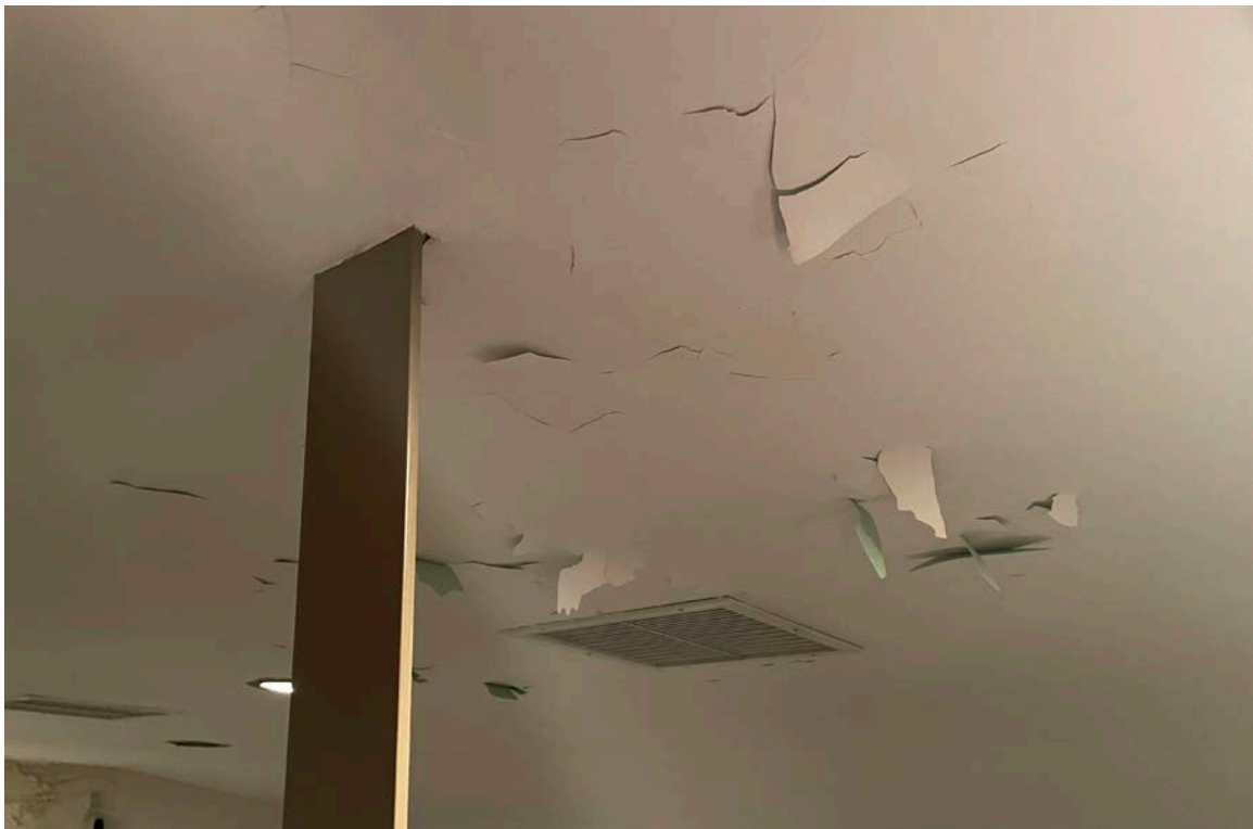
Figure 26: Weldon Auditorium: Detail of ceiling above the catwalk. Note ceiling damage.
