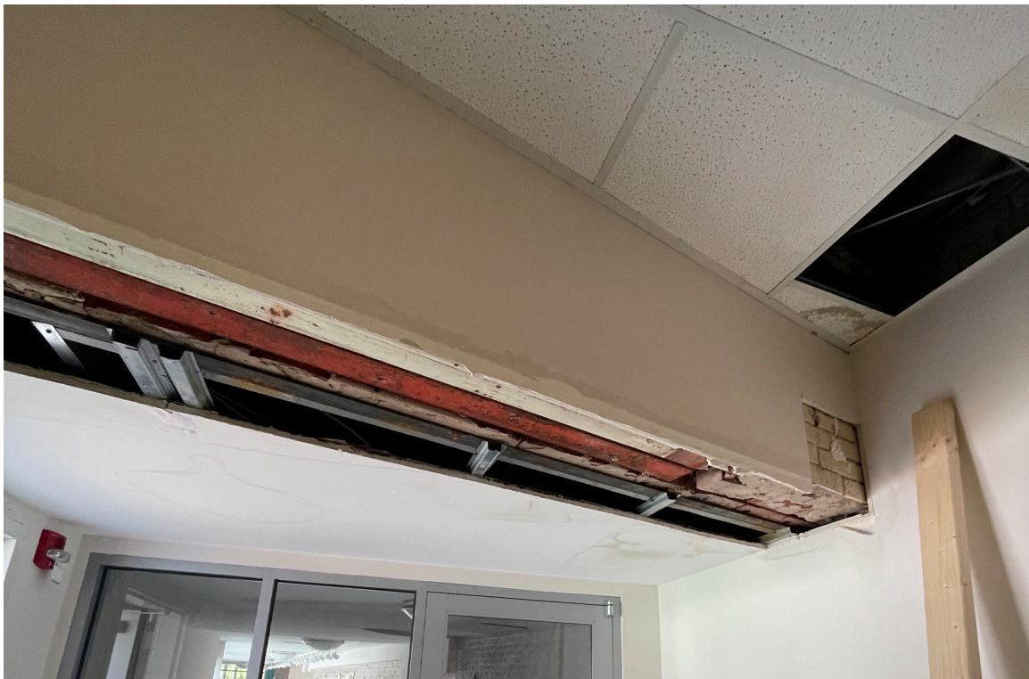
Figure 32: Weldon Auditorium: Detail of masonry following removal of the drywall. The existing steel lintel and masonry were found to be unsupported and were structurally unsafe.
