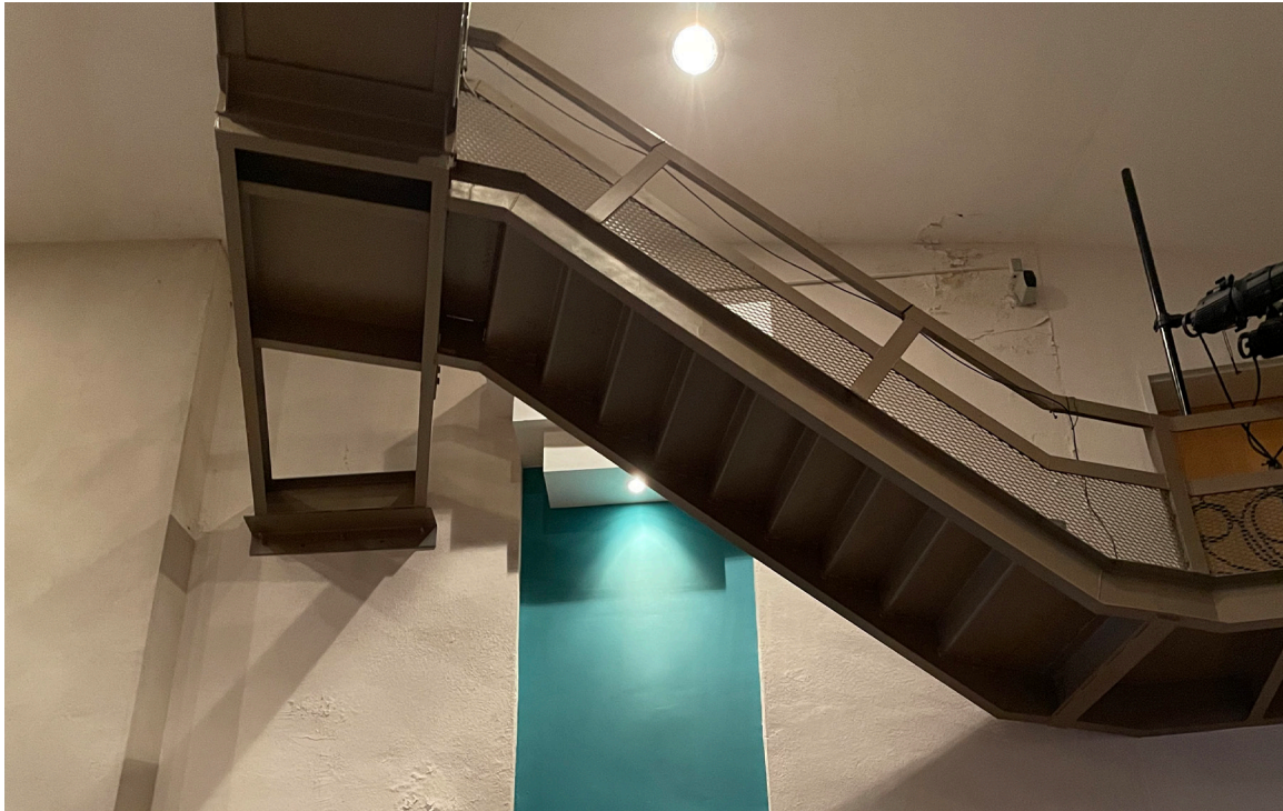
Figure 25: Weldon Auditorium: Overview of the catwalk and ceiling above the stage. Plaster damage is evident along this wall.
