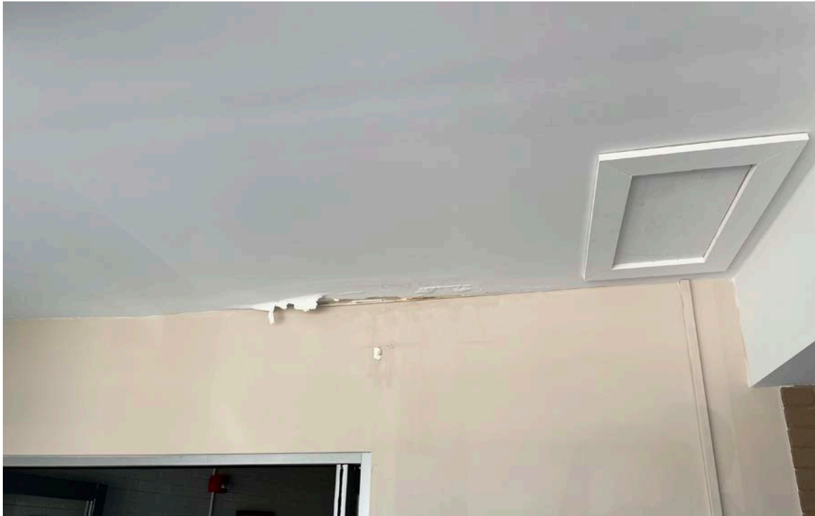
Figure 20: Weldon Auditorium: Hall of fame ceiling damage.
