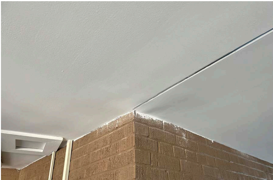
Figure 21: Weldon Auditorium: Damage is present at the intersection of the original auditorium building and the Hall of Fame Addition.
