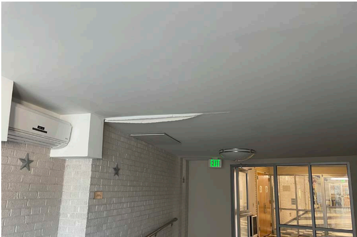
Figure 23: Weldon Auditorium: Detail of drywall tape failure due to moisture intrusion.
