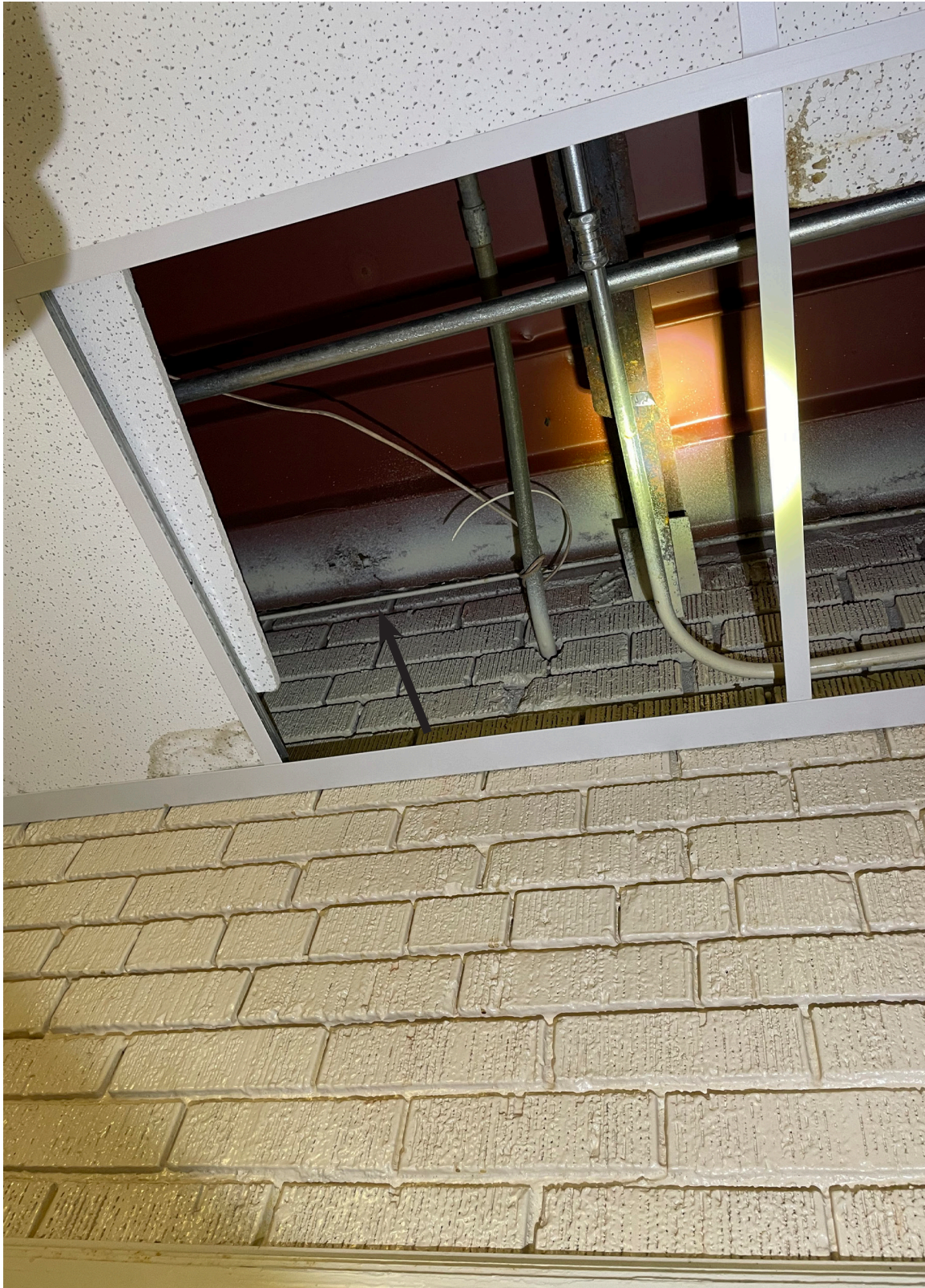
Figure 24: Weldon Auditorium: Detail of corrosion within the decking above the drop tile ceiling.
