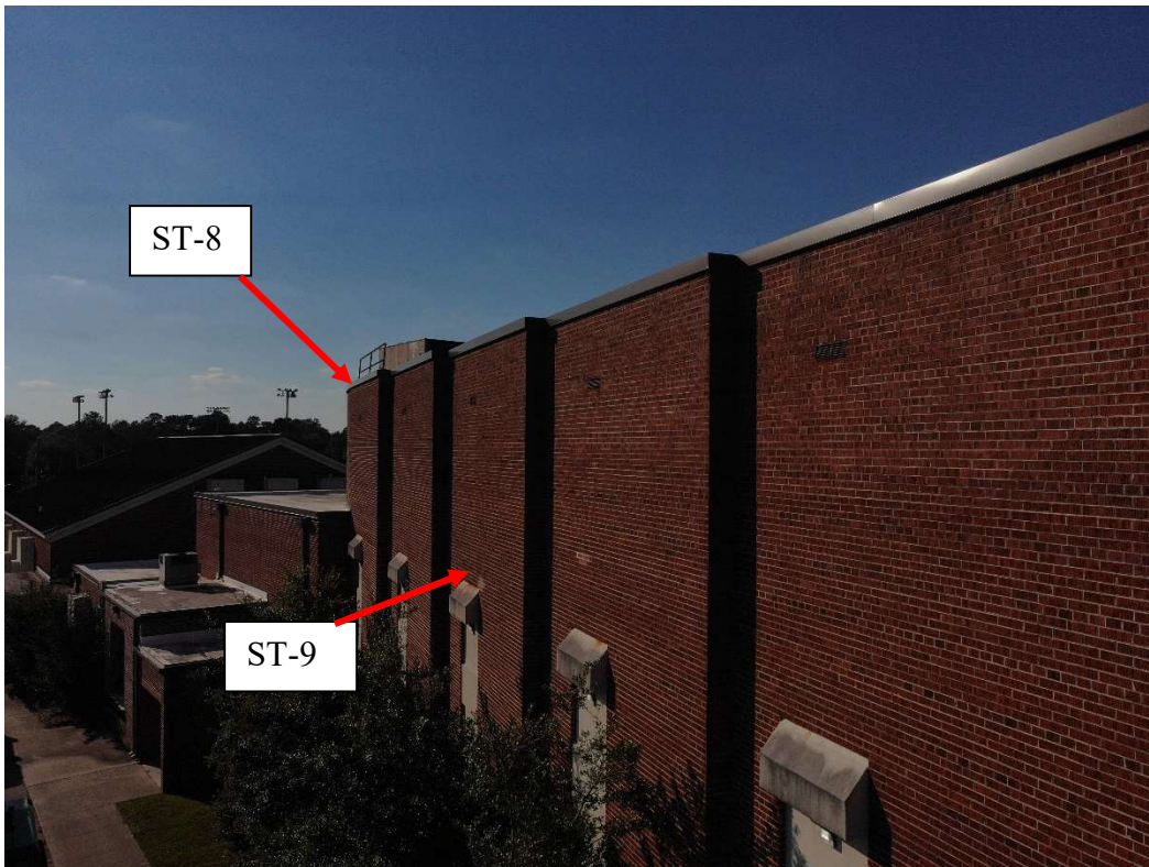
Photo 6: DT & ST locations at R3
