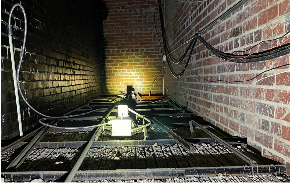
Figure 28: Weldon Auditorium: View above balcony stair ceiling. The exterior masonry wall is at left and has been waterproofed with a black coating. White efflorescence is visible within the mortar joints indicating active water intrusion through the masonry and black coating.
