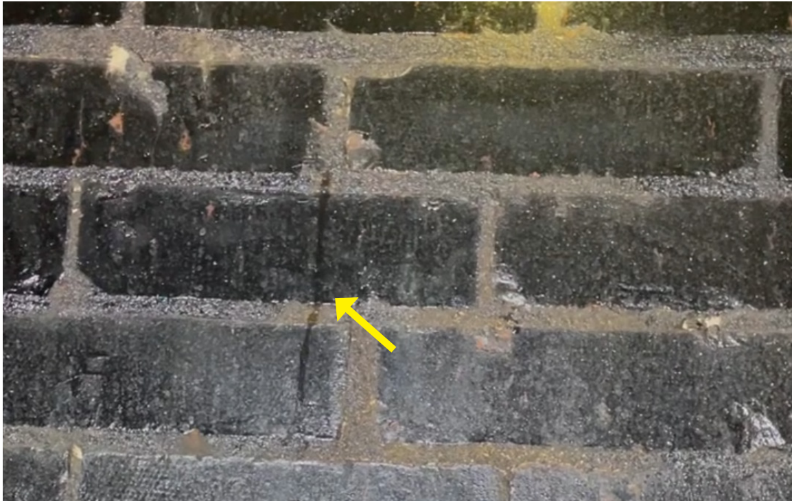
Figure 30: Weldon Auditorium: View of water actively migrating through the masonry above the balcony ceiling (arrow) during the dynamic water testing.
