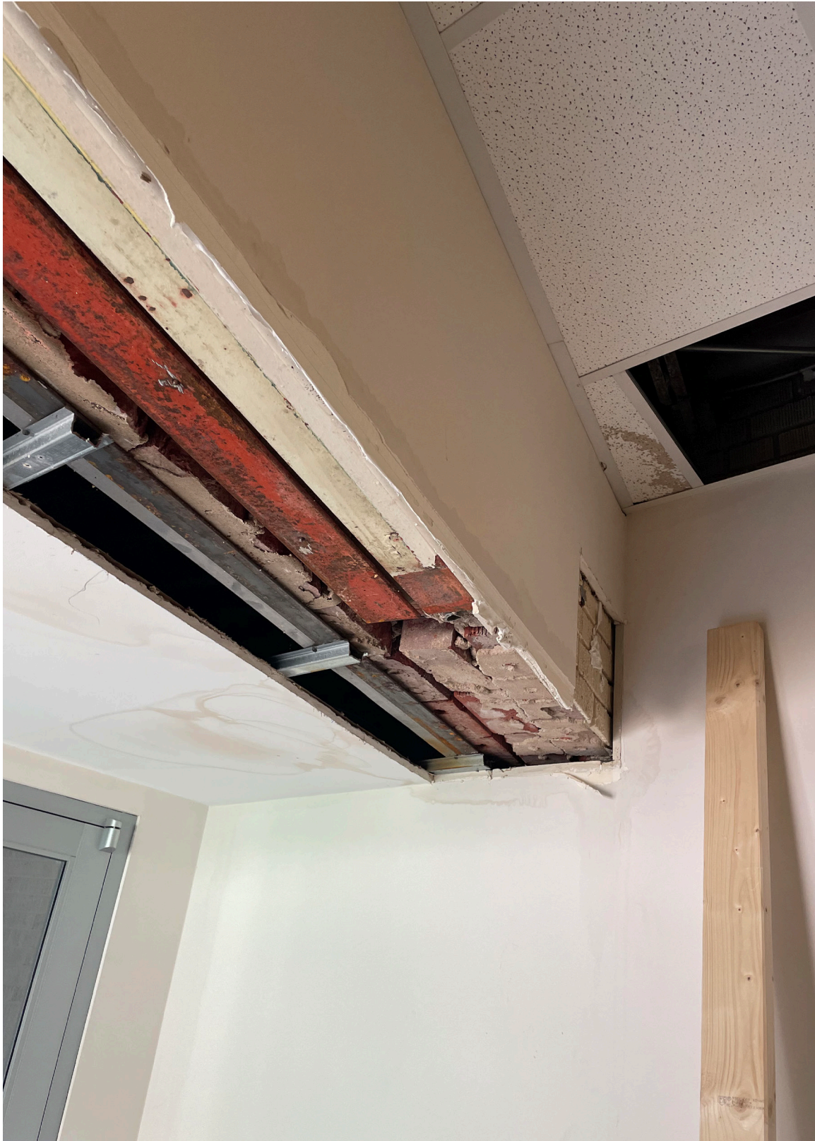
Figure 33: Weldon Auditorium: Additional view of existing orange steel lintel and unsupported masonry.
