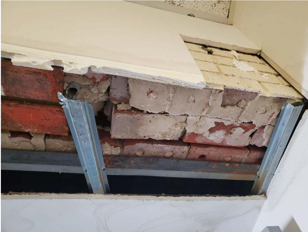
Photo 13: View from below unsupported brick wall at DT-3
