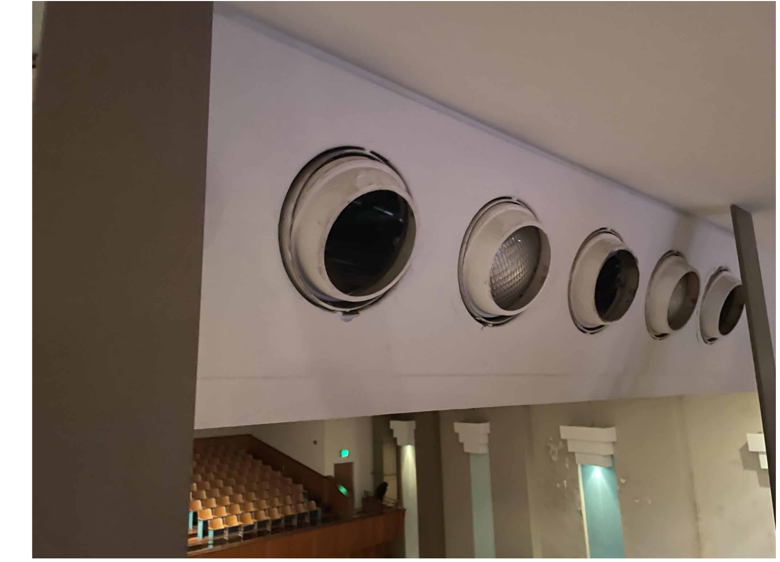
2 UNUSED PENETRATIONS IN AUDITORIUM CEILING 3" = 1'-0"
