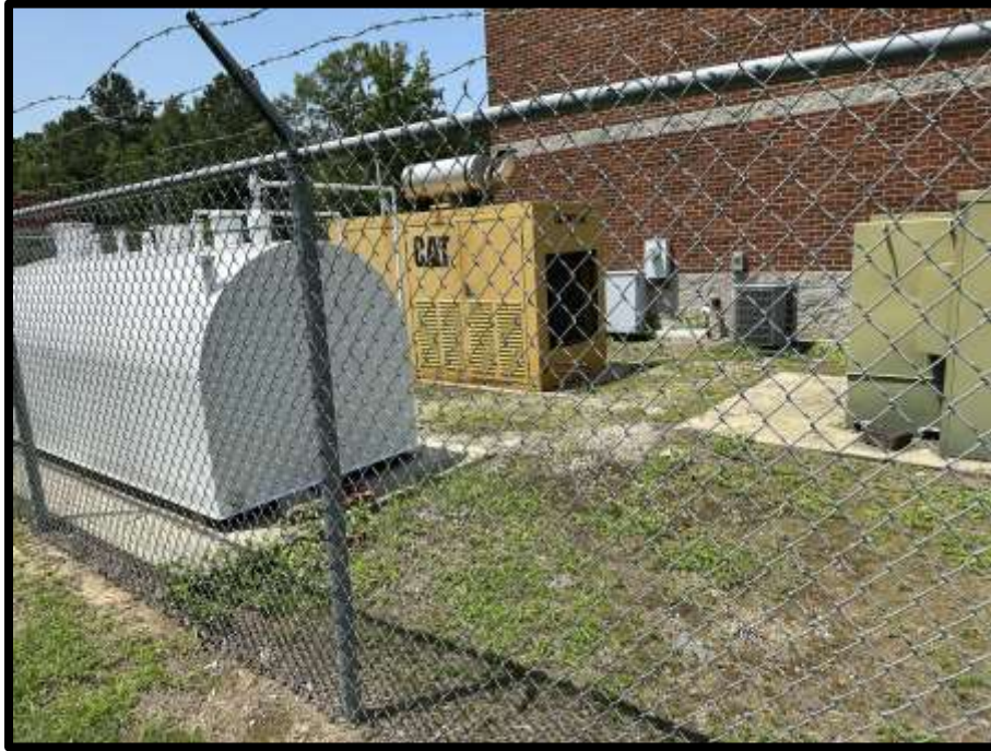
Photograph 1: Generator and Aboveground Storage Tank (AST) near Fire Station.
