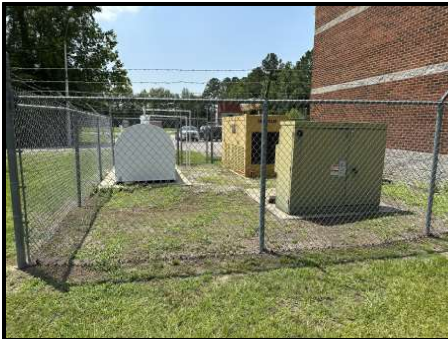
Photograph 4: Generator and AST near Fire Station
